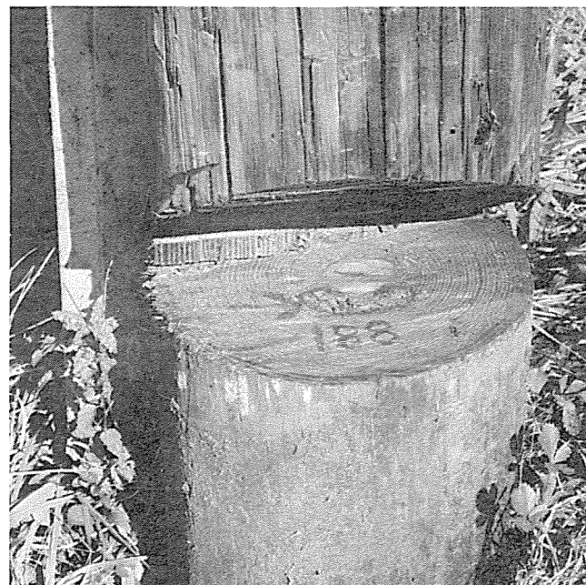
Figure 3. — Closeup of same pole shown in Figure 2, revealing small pocket of internal decay.
